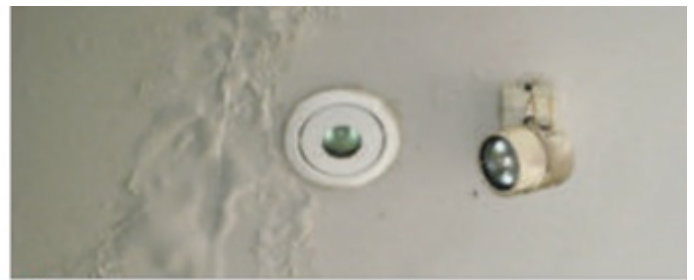
❌ Example: Gypsum Board Not humidity resistant
